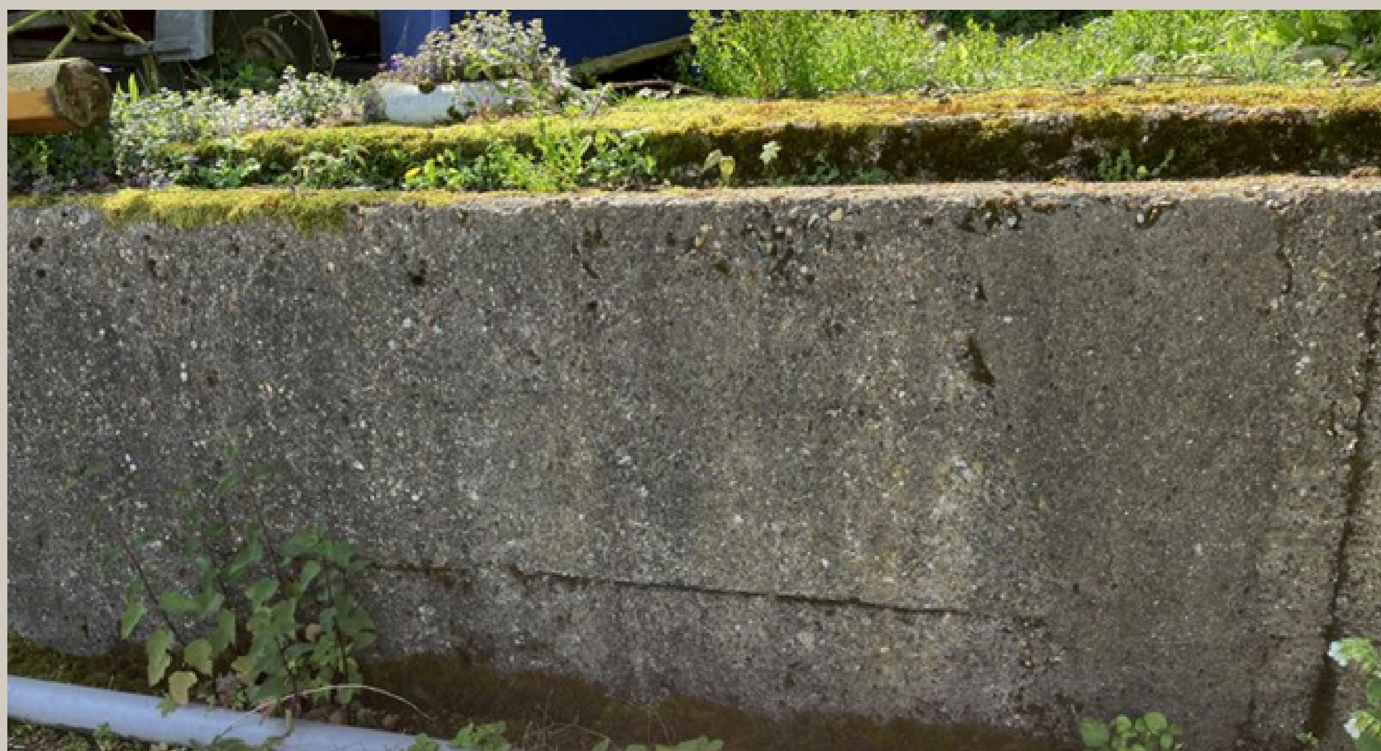
6. Concrete block retaining wall, built of three layers of separate blocks. Each section 30 cm (1ft) high and approx. 6m (6.6 yds) long.
